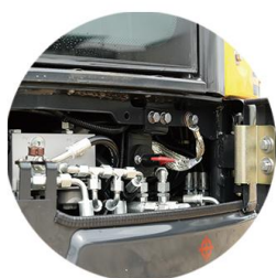
09 Main battery switch
